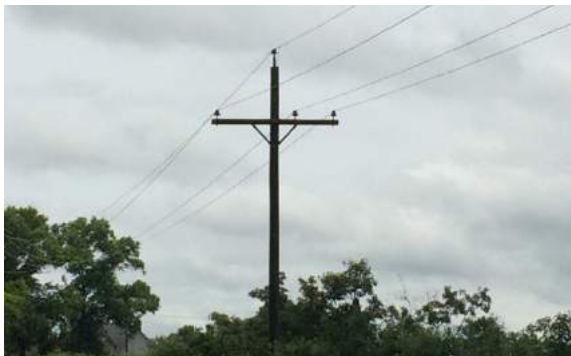
Local power line on E 1200 Rd
