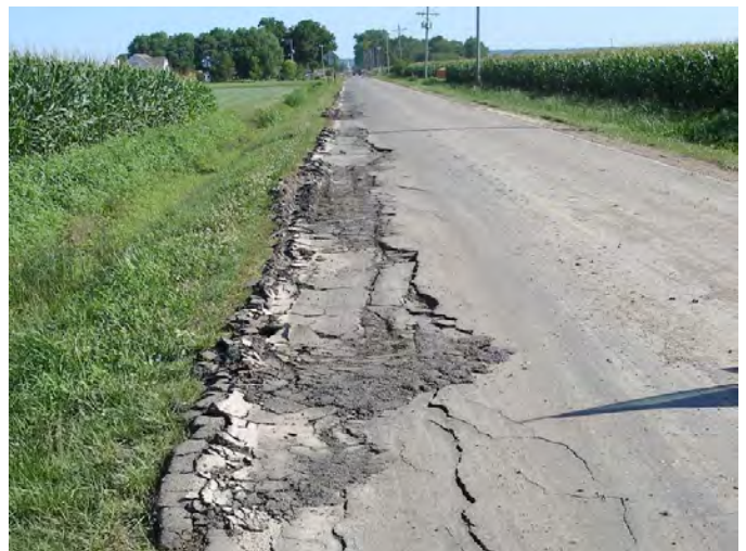
Pavement damage Route 9
