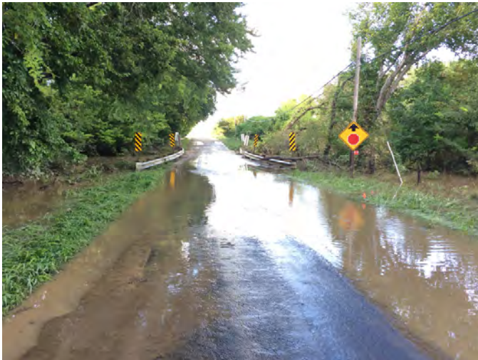
Existing roadway flooded July 2017
