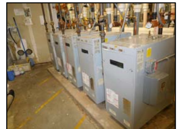
Existing building boilers
