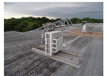
Substantial De-Mineralization on Community Health Building Roof
