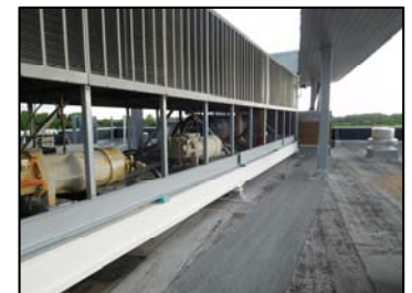
Existing 100-ton chiller
