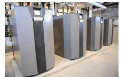
Modern Condensing Boiler With Higher turndown
