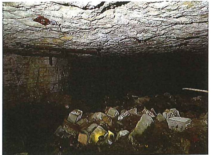
Void from Caves Under Site - Roeland Park, KS
