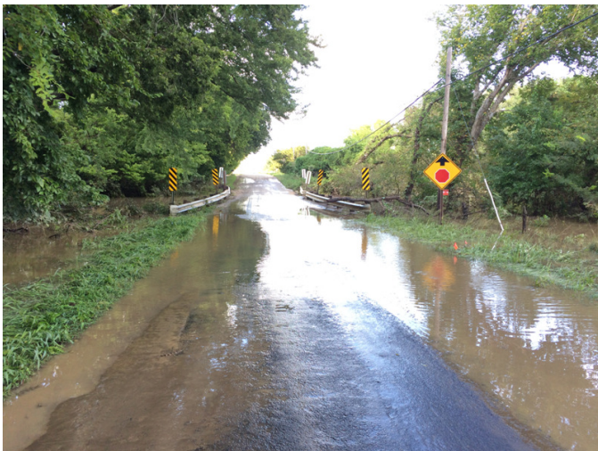
Existing roadway flooded July 2017
