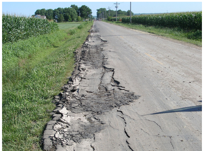
Pavement damage Route 9
