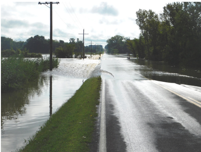
N 1000 RD flooded July 2017
