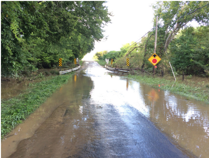
Existing roadway flooded July 2017
