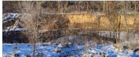
Bank erosion and Scour
